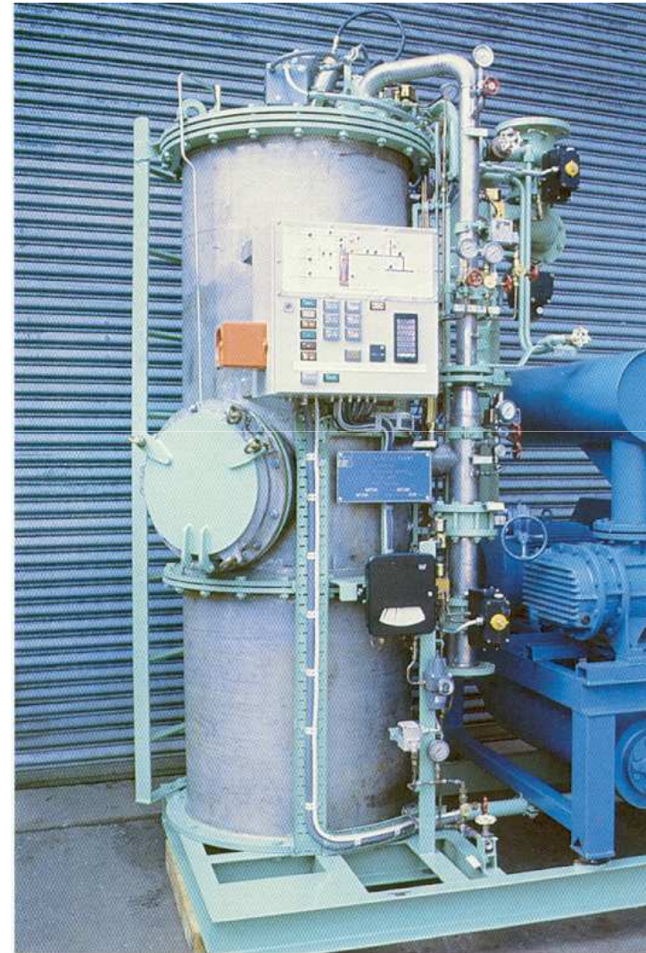
The burner/scrubber unit
